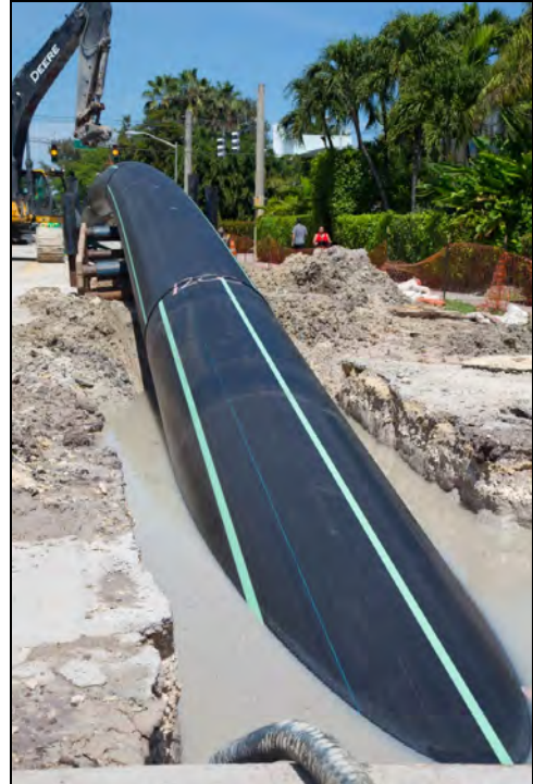
The fused HDPE pipe entering the pit. More than 3,300 feet of 54-inch diameter HDPE pipe was used.
