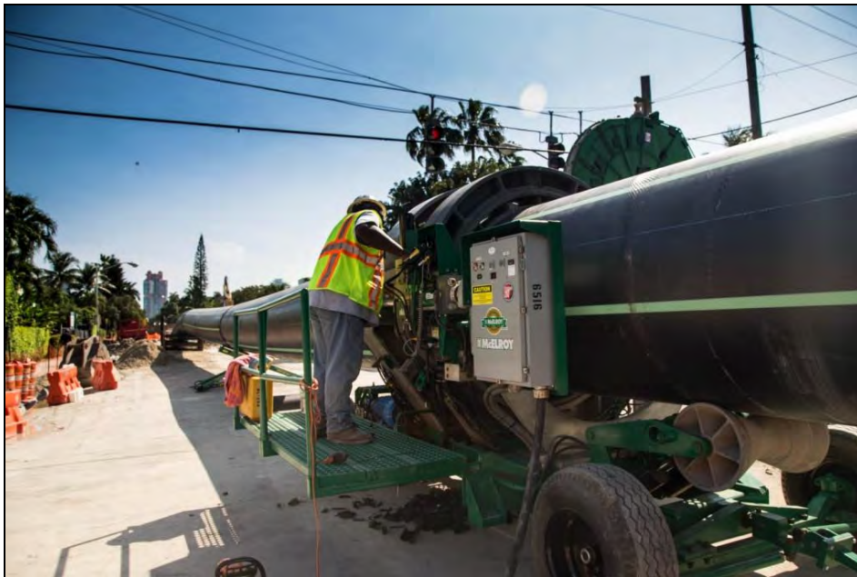
An ISCO field tech used a McElroy 2065 fusion machine to make the final tie in.
